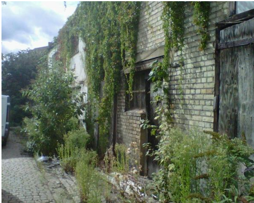
Image 1: View of existing derelict buildings at the site looking along the Mews in SE direction.
